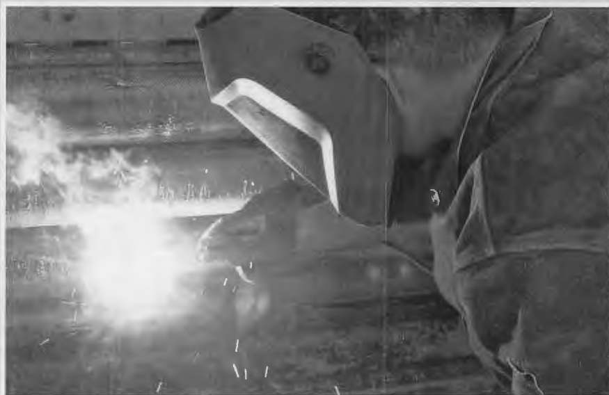
Spc. Greg Knauff, from the Arizona Army National Guard, welds a piece of metal over a hole in the fence along U.S./Mexico border near San Luis, Ariz. This photo appeared on www.army.mil .
